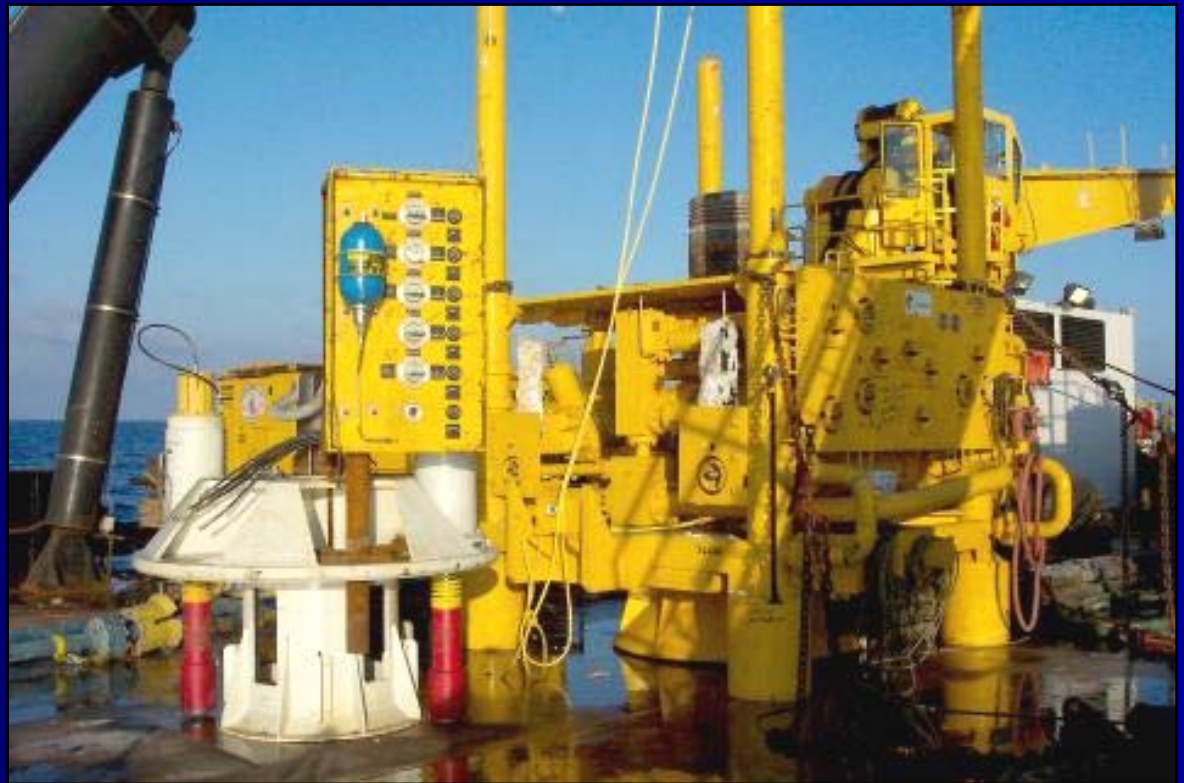
Tree Retrieval Tool with ROV Panel (left of tree #3) allows unlatching and pulling of the tree on cable.
