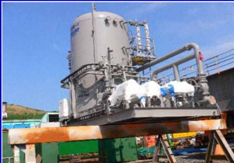
Gas Flotation Skid
