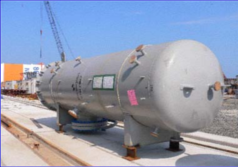
Crude Run Tank
