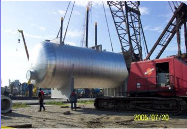
Oil Treater Vessel
